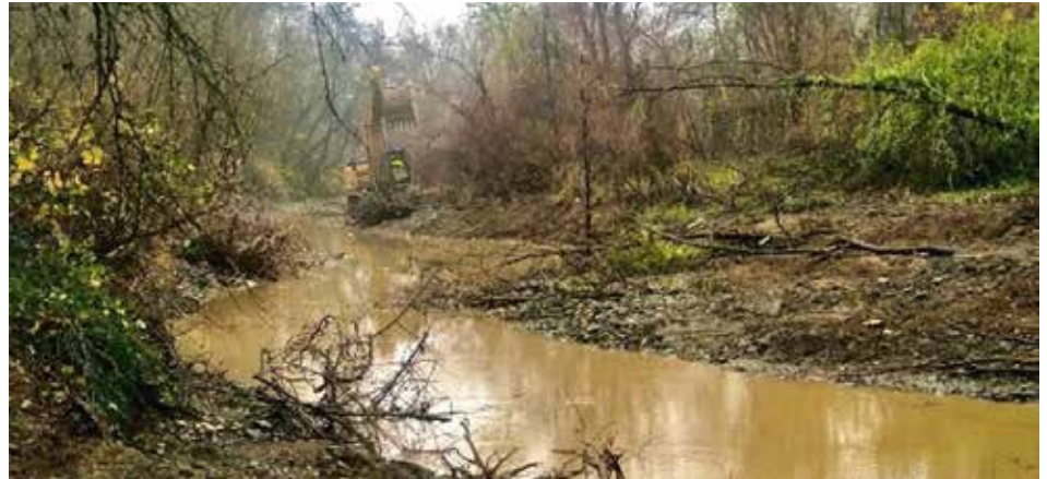
Anderson River Park side channel restoration is back on track thanks to GSSA intercession
